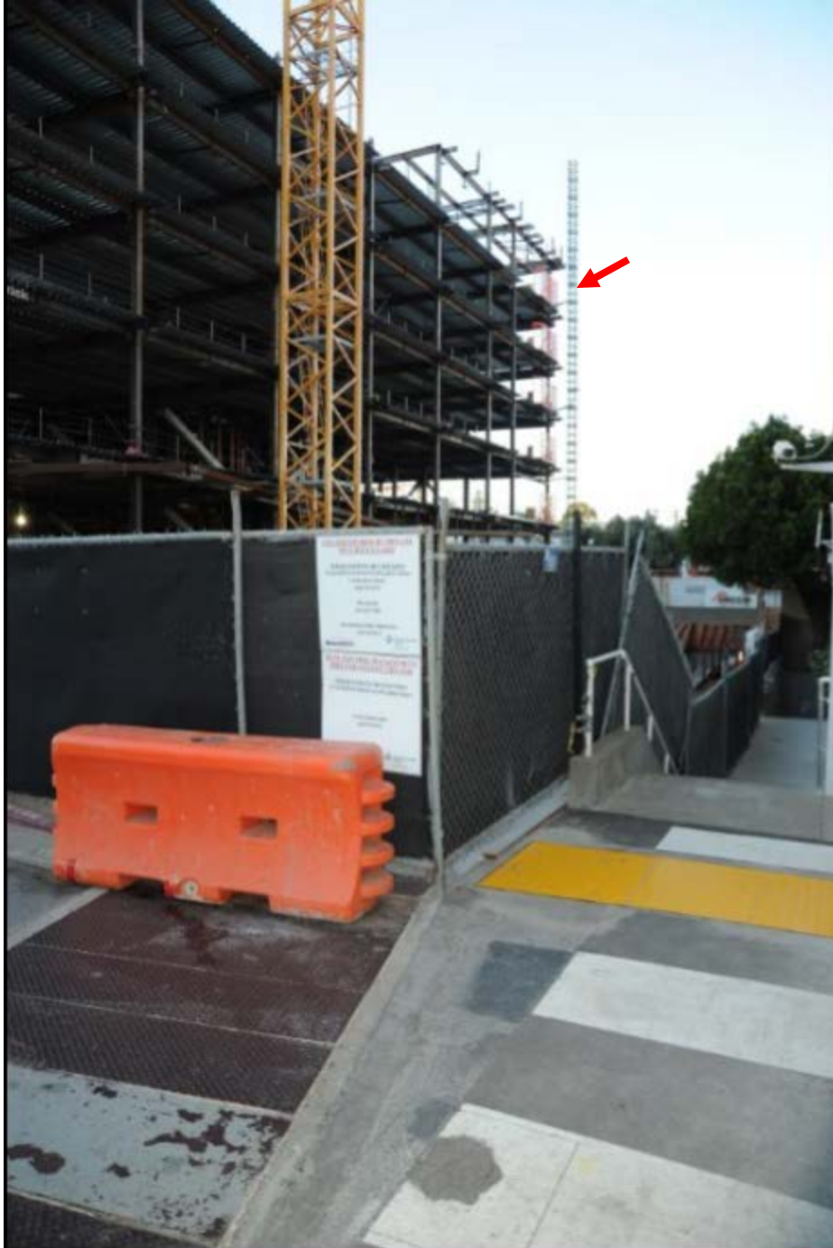
Figure 3: Depicts approximate vantage point of Officers Garza and Stokes. Tall tower structure in the distance is the manlift shaft. Note, although the manlift shaft is visible in this photo, the actual manlift is not. Red arrow indicates Lopez Garcia's approximate location at the time of the incident, although, again, the actual manlift he stood on top of is not shown (Source: SFPD).
