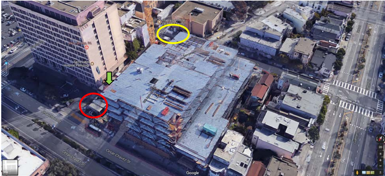
Figure 1: Site of incident. Green arrow indicates Lopez Garcia’s approximate position atop a manlift at the sixth floor (actual manlift not shown). Yellow oval represents approximately where Officers Stokes and Garza were positioned at the southeast corner of the construction site. Red oval represents where Officers Suhrke and Camilosa, and Sgt. Aloise were positioned at the northeast corner of the construction site. (Source: Google Maps).
