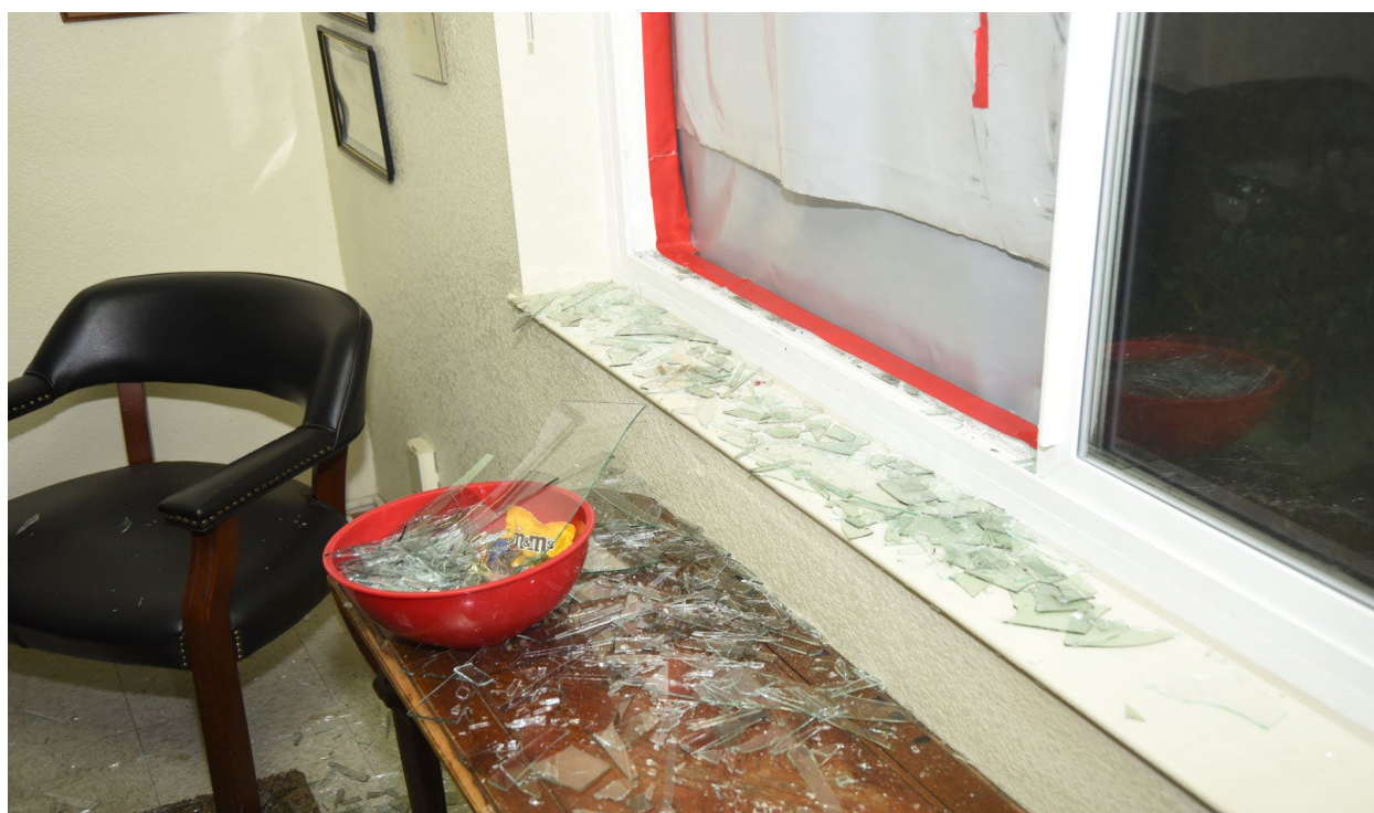
Figure 22-Damage to the interior of the leasing office unit at 1433 F Halibut Court and broken window.
