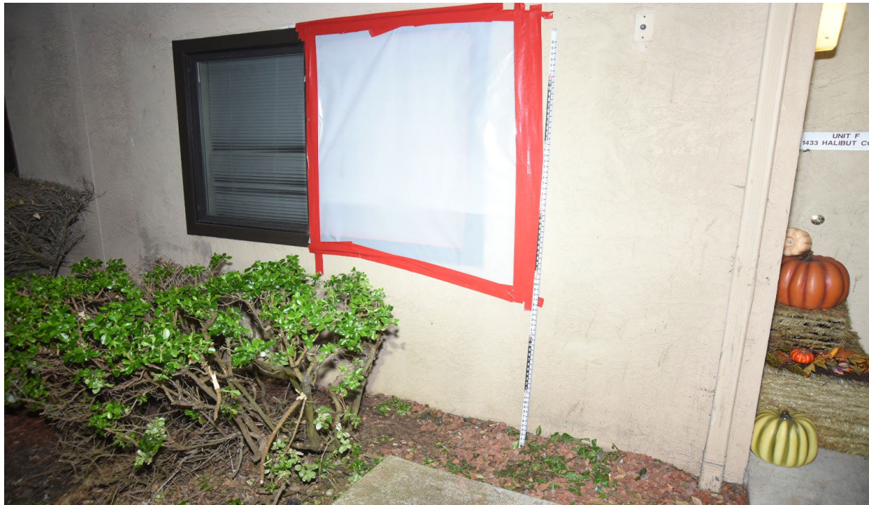
Figure 20-View from outside of the leasing office unit at 1433 F Halibut Court and the damaged window taped by SFFD.
