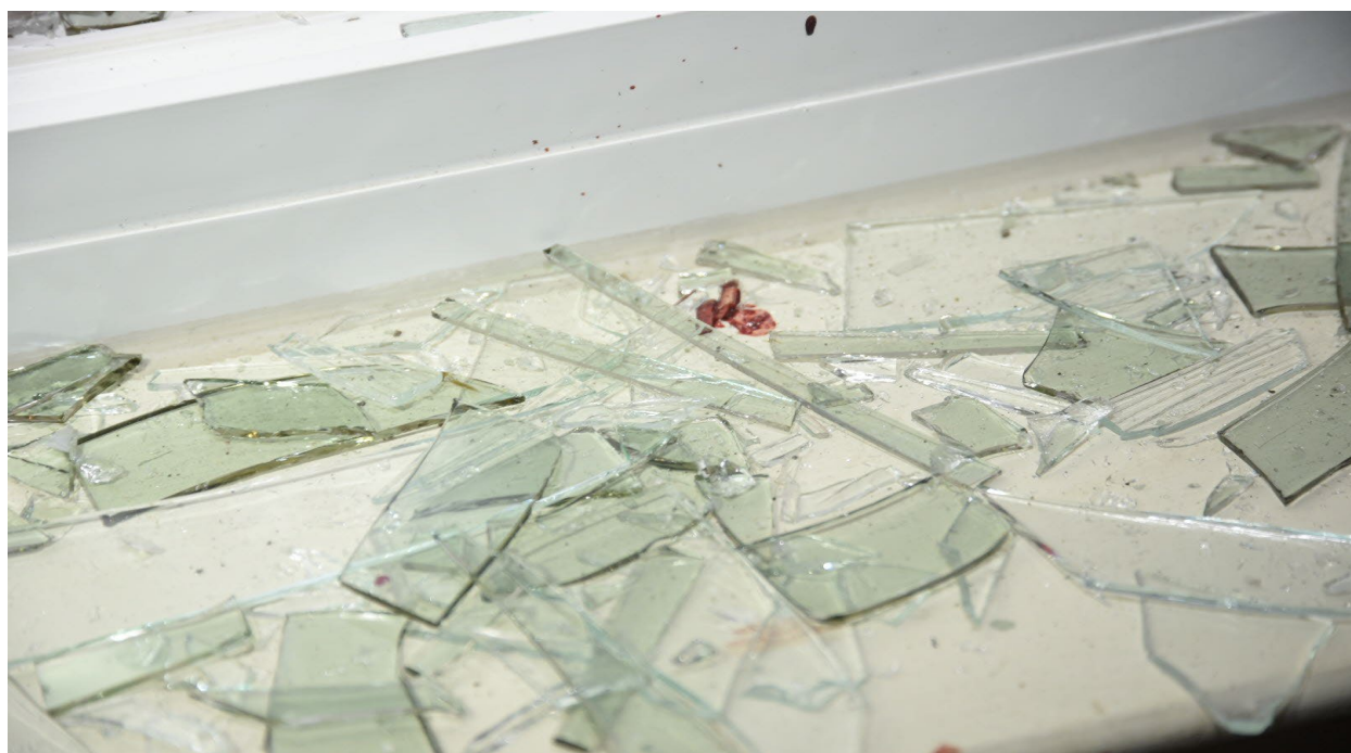
Figure 23-Broken glass and a close-up perspective of the damaged interior of the leasing office unit at 1433 F Halibut Court with a red substance later confirmed to be blood.
