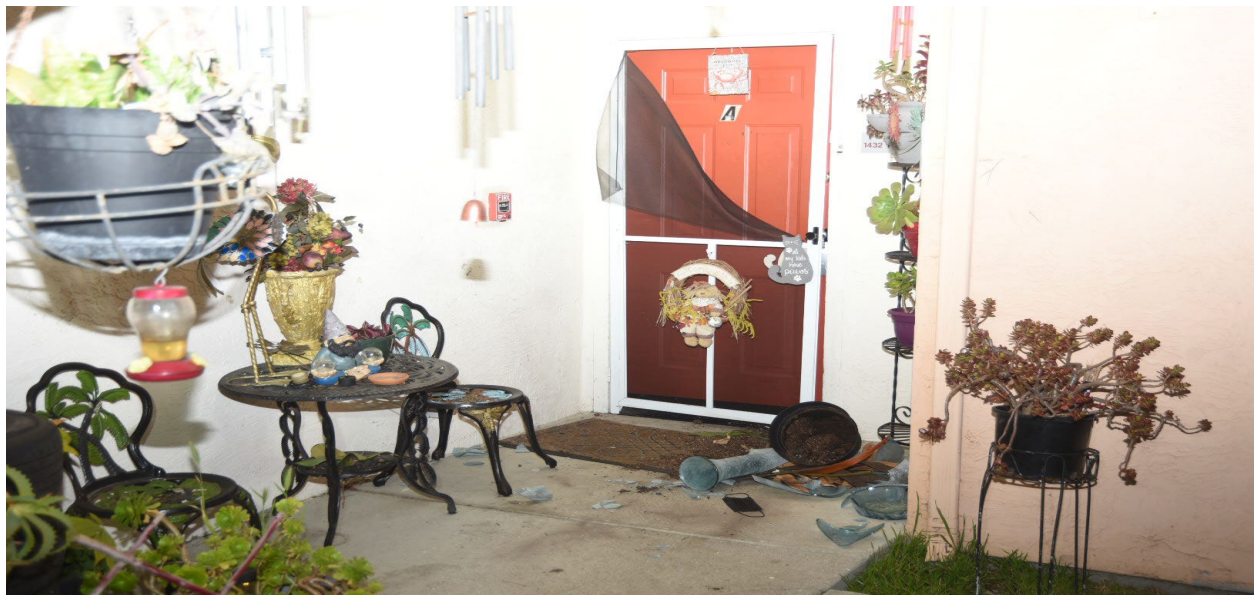
Figure 2- Front door of V-1's apartment unit (1432 A Halibut Court) and visible damage.
