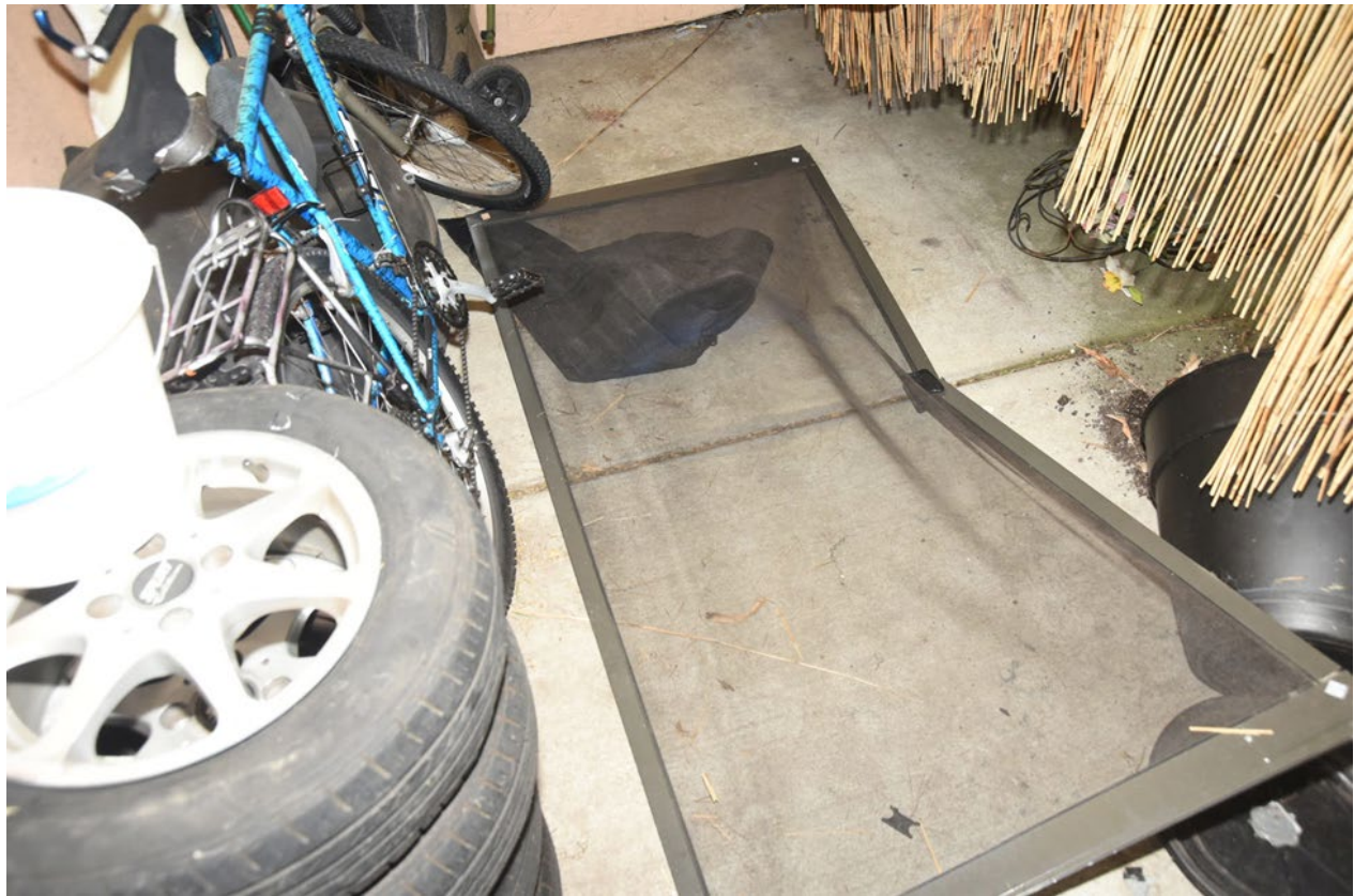
Figure 6- The back patio area of 1432 A Halibut Court with a closer view of visible damage to the rear patio screen door.
