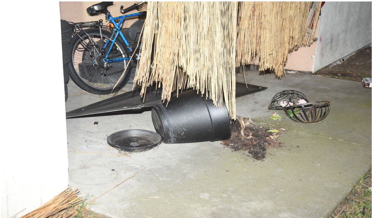
Figure 5- View of the back door of V-1's apartment and patio area of 1432 A Halibut Court with visible damage.
