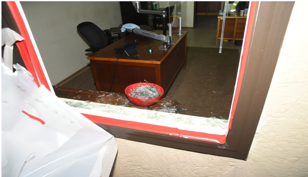
Figure 21-Damage to the interior of the leasing office unit at 1433 F Halibut Court and the damaged window looking into the office area.
